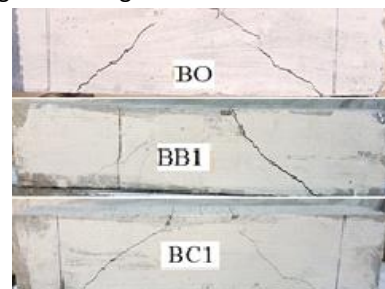
Fig. 10 Crack patterns for all beams
